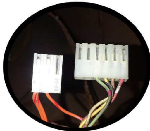
Photo: 3 and 6 pin video signal connectors disconnected.
